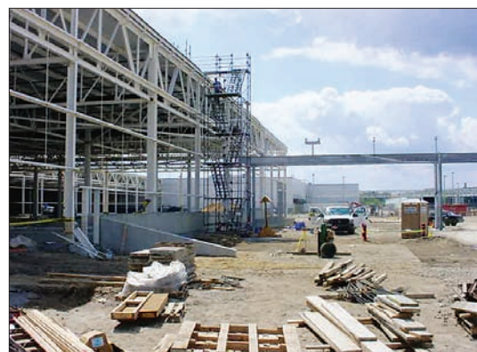
▲ V6. Comprehensive 3-D modeling cuts clutter and activity on site. Parts arrive cut to fit. No trash, no dumpsters.
