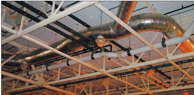
▲ Tight. Trimming on site is one thing, pre-fab to perfection is another.
